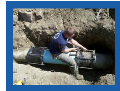
Photo on the left shows Operator I, Barry Silva, straddling 12" water main during repair.
